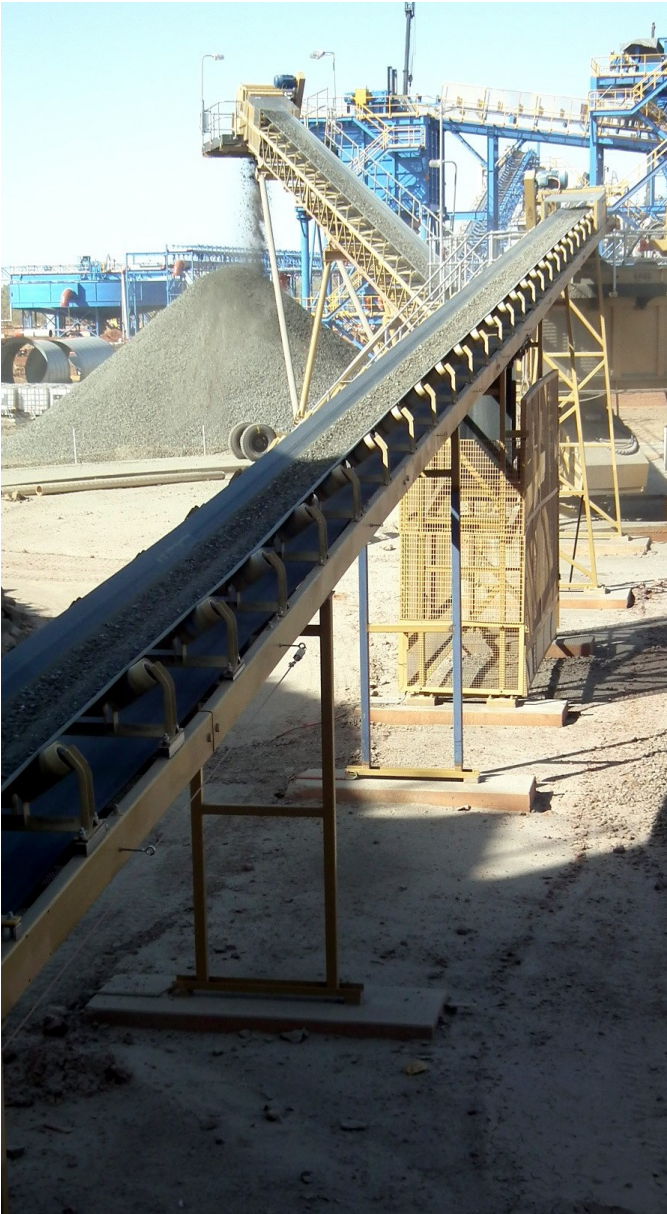
Figure 4: Conveying Screen 1 ore product to the crushed ore stockpile, which feeds to the main Processing Plant via the underground reclaim feeders
