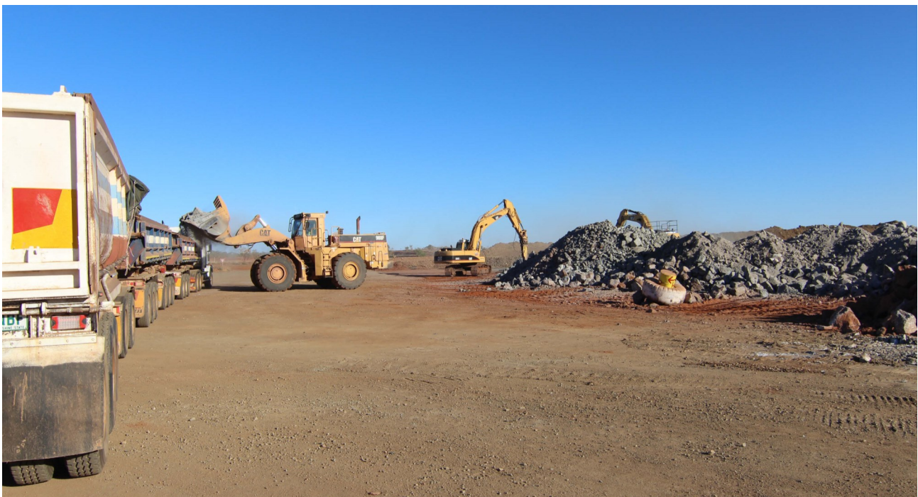
Figure 8: Contractor loading road trains with Rocklands primary ore ready for shipment to EHM processing plant
