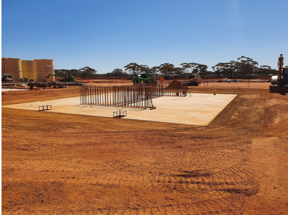
Kiln pad and pier under construction to enable delivery of the kiln shell
