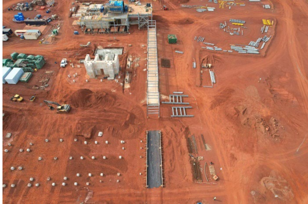
Image 8 - Wet plant and pipe rack
