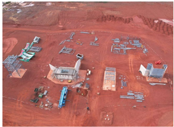
Image 5 - Fine ore bin and reclaim area
