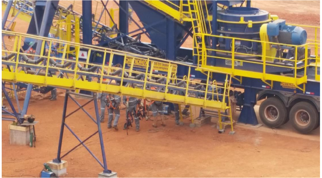
Secondary cone crusher/screen of local manufacture, being configured to produce a -20mm sized feed to the ball mill. The ball mill feed will be stockpiled above the reclaim tunnel below
