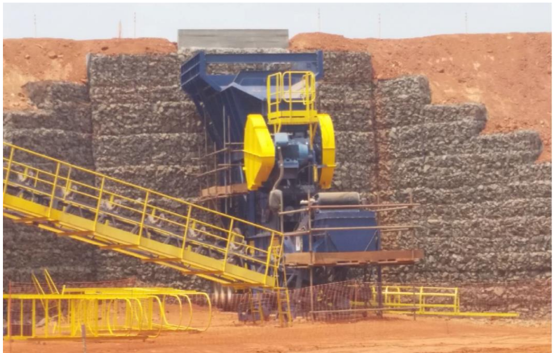
Earthworks associated with the initial ROM Pad construction have been completed and the retaining wall erected. The jaw crusher has been installed below the tip head – awaiting only the feed hopper, grizzly and electrics
