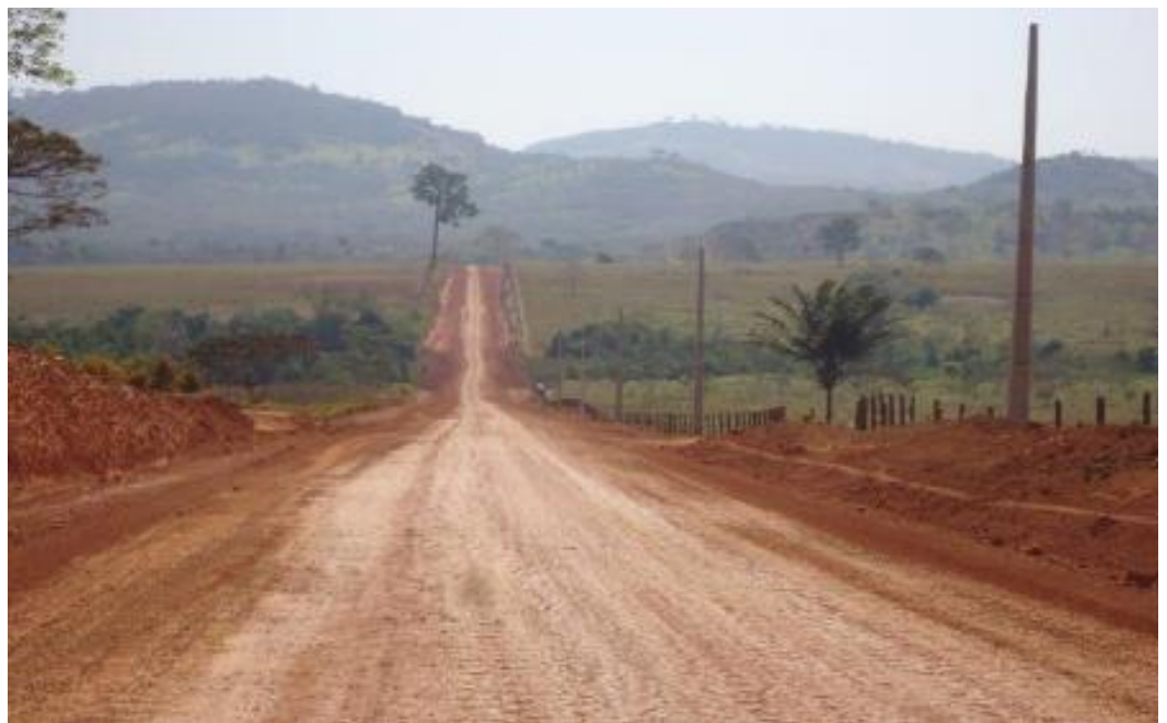
The mine access road including construction of a number of river bridges is ongoing. These are expected to complete before the wet season
