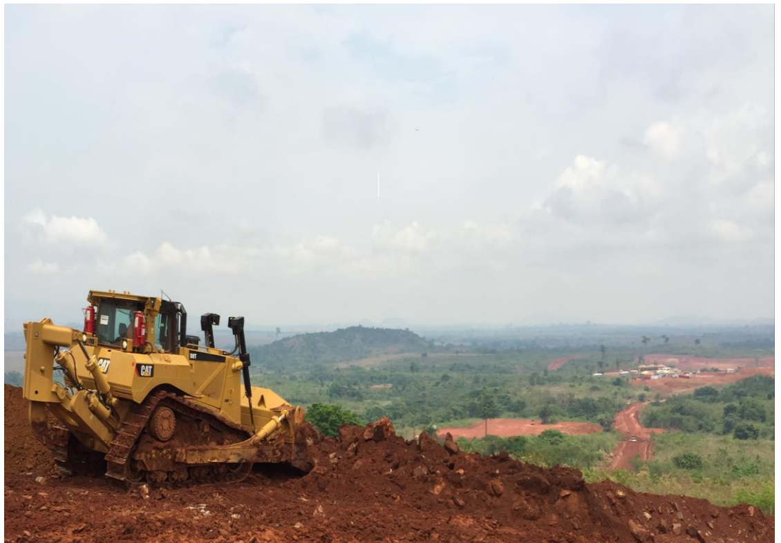
MACA's D8 Dozer pushing the haul road forward toward the plant in the distance
