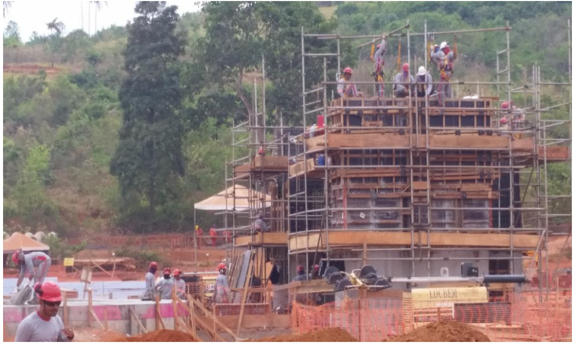
Installation of the Ball Mill concrete foundation represents the most complex civil works of the project. This activity has now reached the trunnion pedestal elevations where precision is paramount
