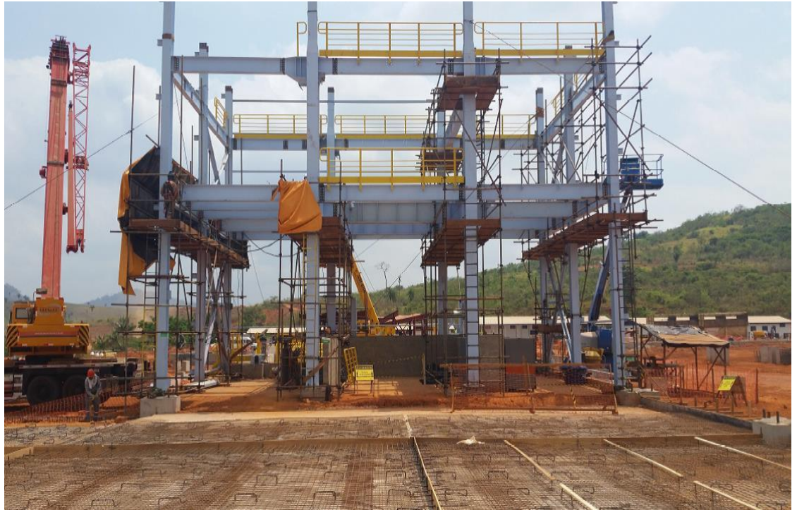
Filter House building footings are completed and structural steel erection building is progressing on schedule
