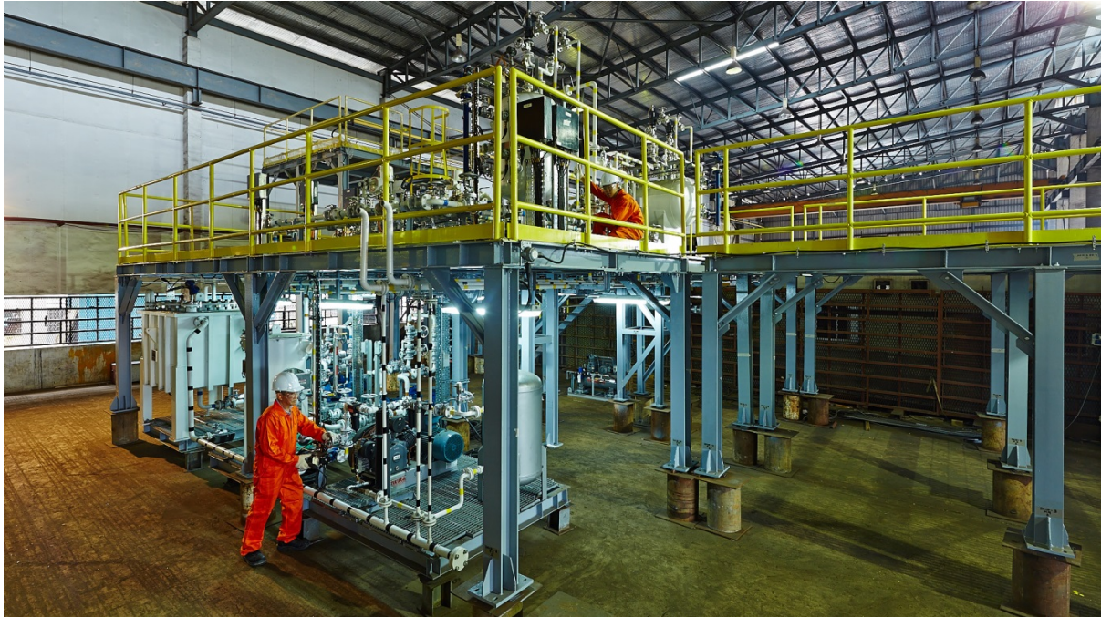
Photo: SGI Energy ‘Safe Live Plant Environment’ in commissioning prior to delivery.
