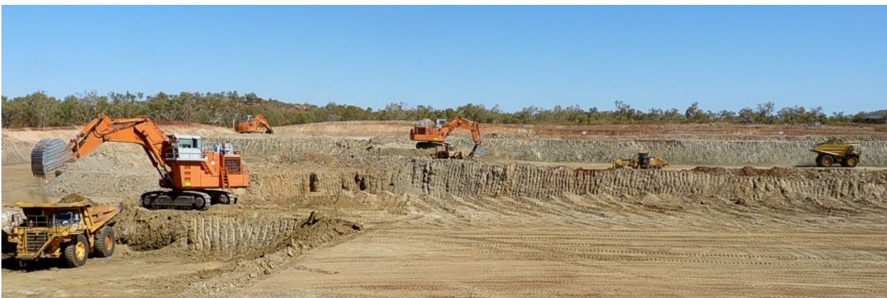
Figure 12: Activity in the middle of the Las Minerale Starter Pit. Waste on flanks of the main ore zones being mined. The previously mined box-cut is in the middle ground between the two diggers.
