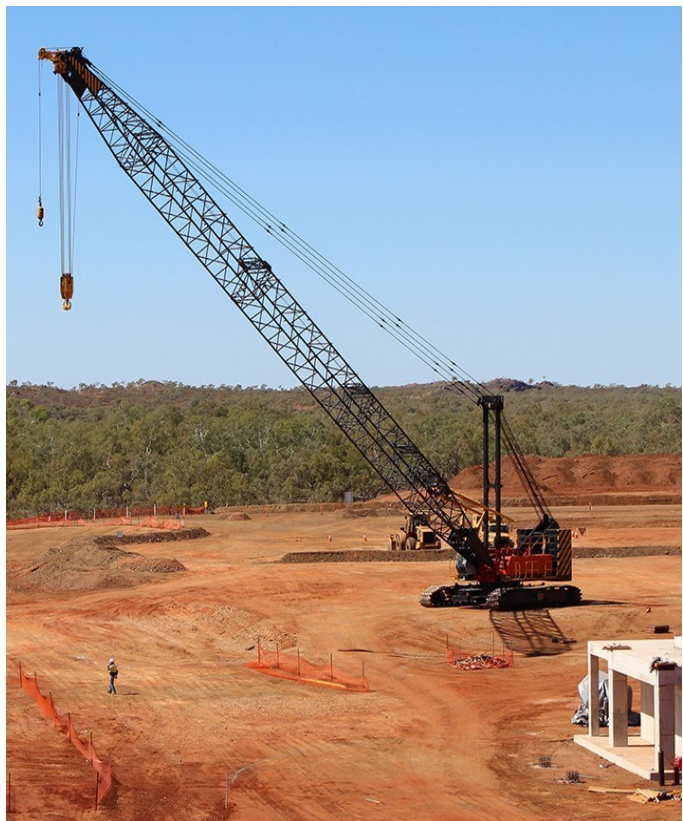
Figure 8: Two Walz 250 tonne heavy-lift crawler cranes have been delivered to site for upcoming major component lifts, such as ball mill, native copper cleaner and various large single-part components. Nine cranes of various lifting capacities will be used during construction.
