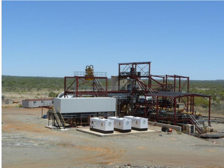
Lorena Concentrator Plant
