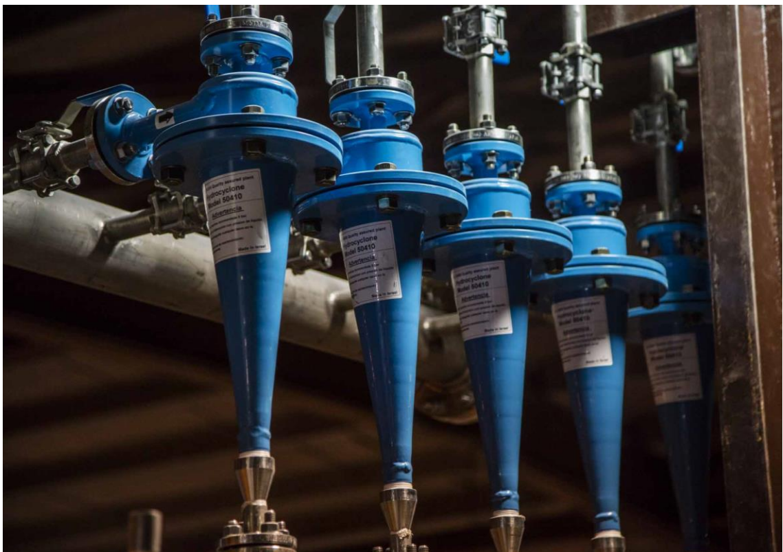
Hydrocyclones installed at Olaroz Lithium Facility
