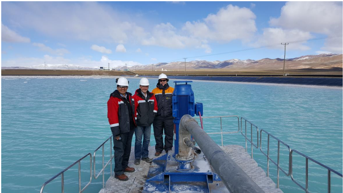
New pontoon based pump recently installed to provide better brine movement control (19 April, 2017)
