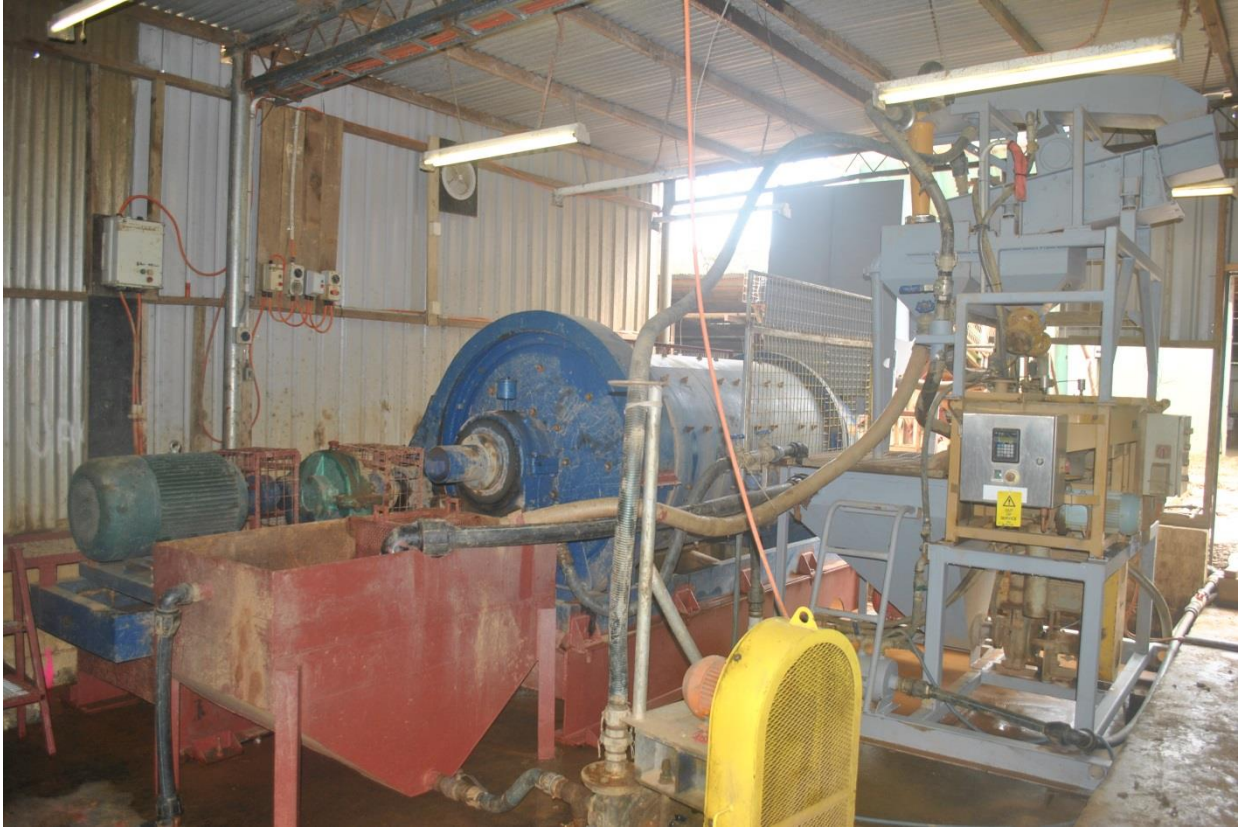
Newly installed 5 tph ball mill and concentrator
