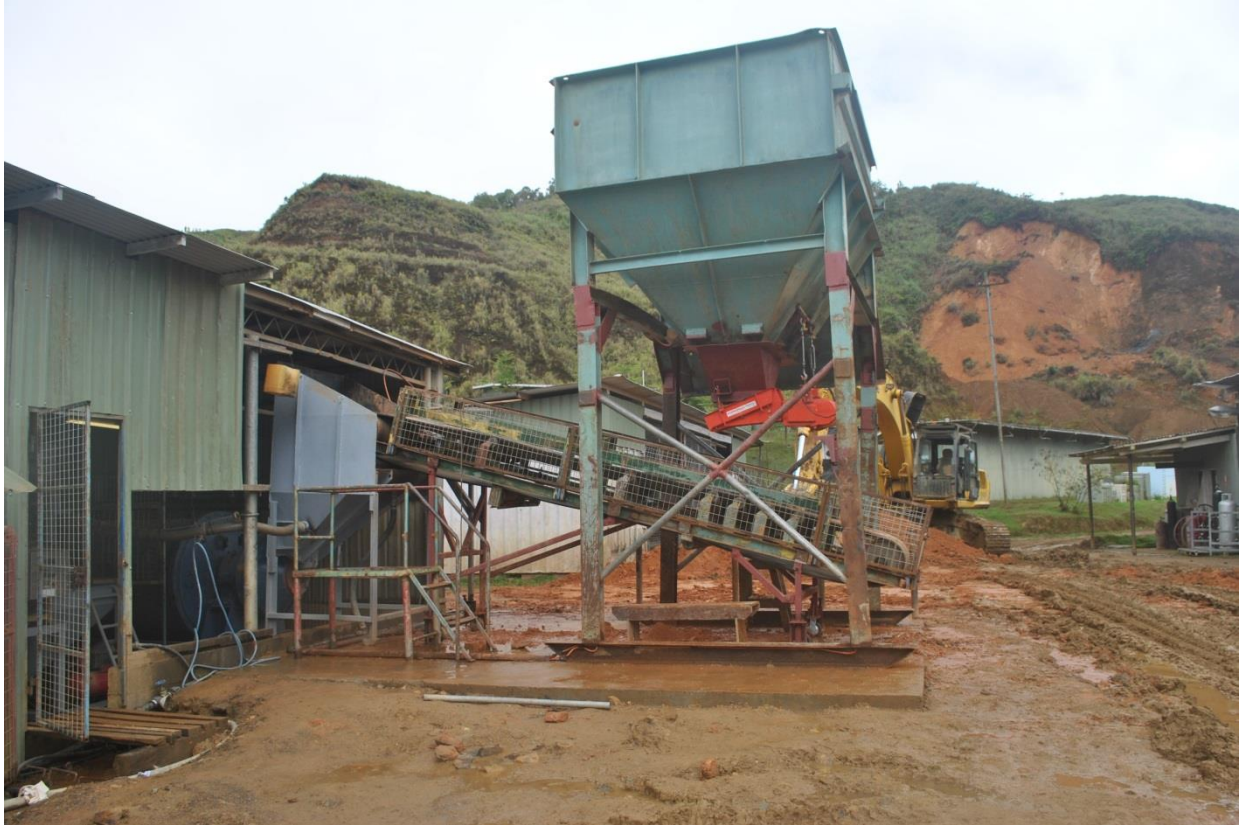
Newly installed mechanical ball mill feeding plant
