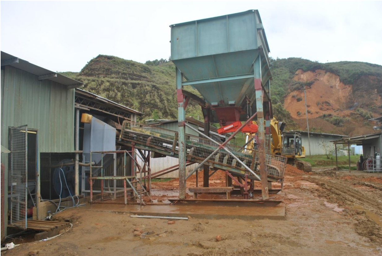
Newly installed mechanical ball mill feeding plant
