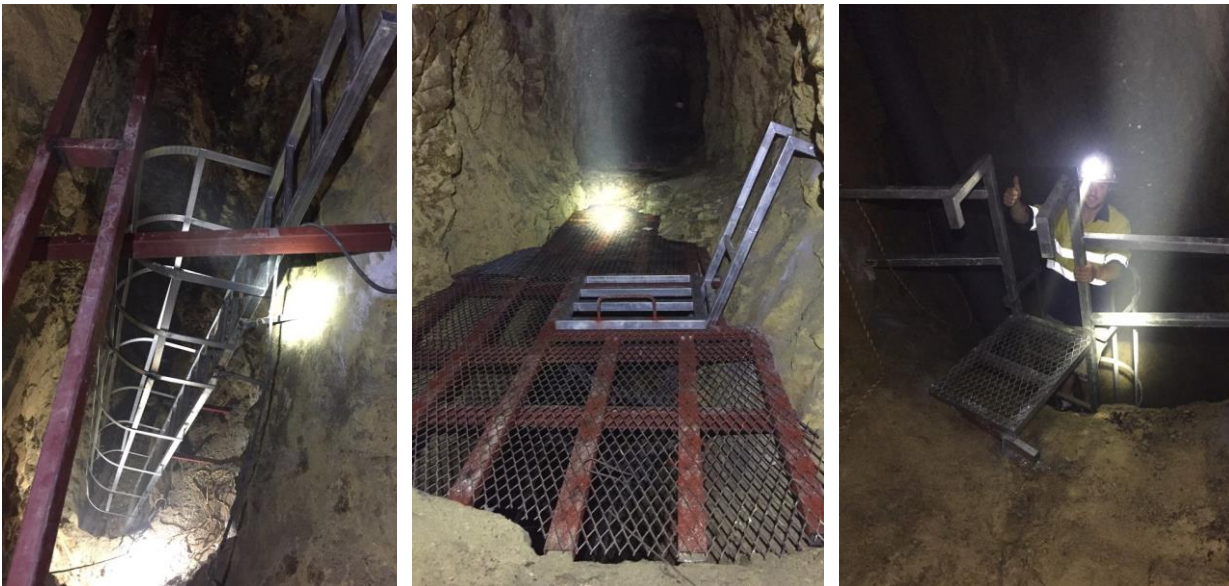
Photos 5, 6 and 7: Weolyu sublevel platform and access with Top level ladder way access at 325mRL.
