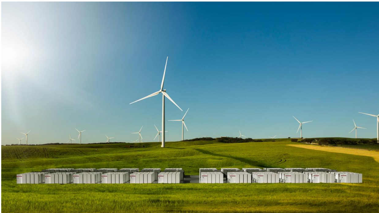
Jamestown Tesla battery farm depiction (source: https://www.tesla.com/en_AU/blog/tesla-powerpack-enable-large-scale-sustainable-energy-south-australia%20 )
