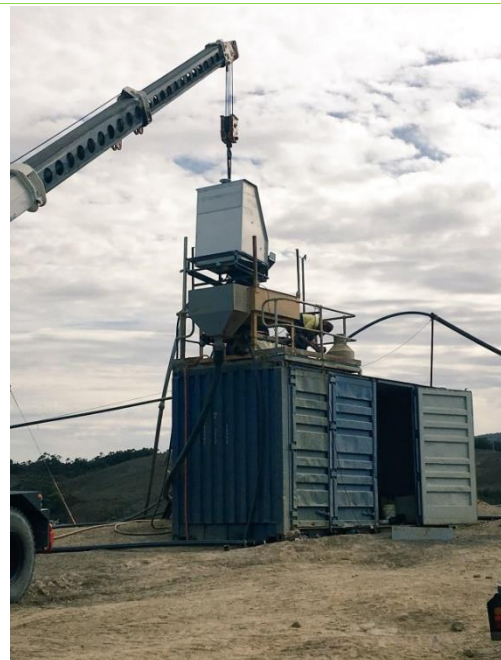
Figure 1b - DSM screen being installed prior to jig to improve tin recovery
