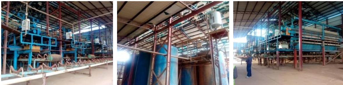
Figure 7, 8 and 9: The Luapula Processing Facility Leaching and Leach Filter Sections
