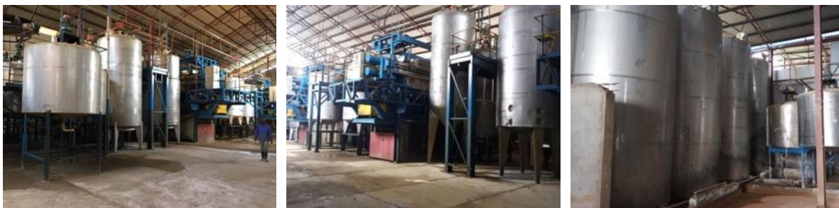
Figure 10, 11 and 12: The Luapula Processing Facility Precipitation Section
