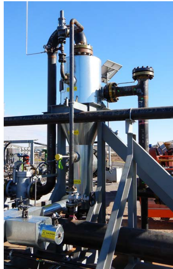
Knock Out Pot (a cyclone that collects and separates water and impurities from Syngas)
