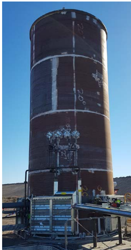
Thermal Oxidiser (processes Syngas and water from Separator Vessel)
