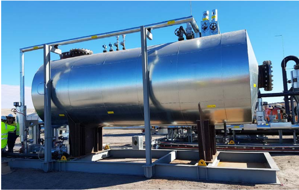
Separator vessel (stores water and impurities from Knock Out Pot)
