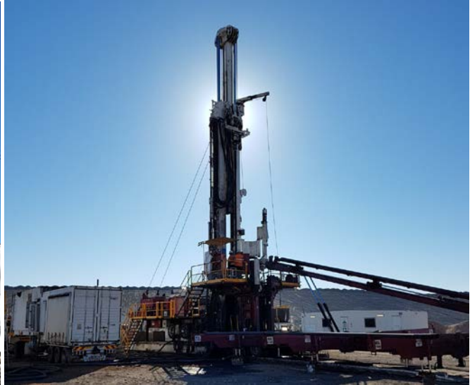
Drill rig installing Inlet Well – generator truck on left, rig with rod handler (red ramp)
