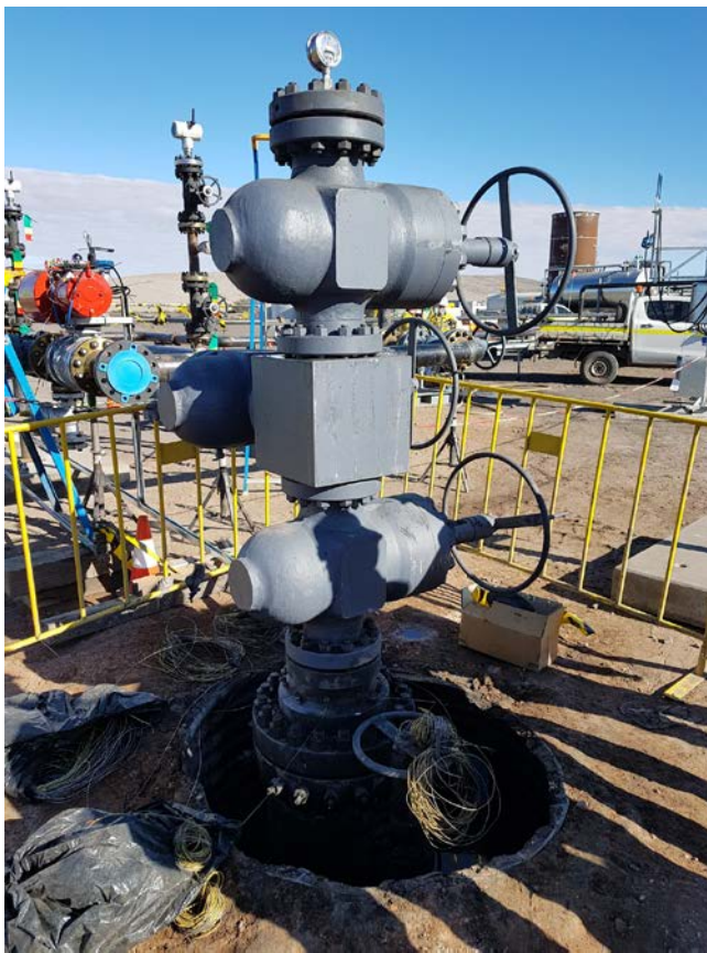
Outlet Well Head, ready for final connection to gas plant. Thermocouple cables at bottom ready for connection to instrumentation
