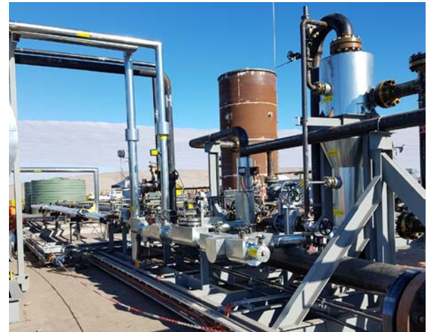
PCD gas skid with valves, instruments and piping
