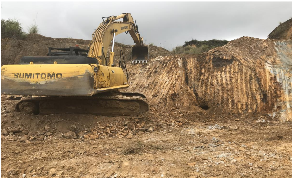
Cutting back the bench to expose the main Edie Lode at the top of Alpha West. The black hole to the right of the excavator, near the left hand edge of the main vein, is an old mine shaft from the earlier 1930s workings.
