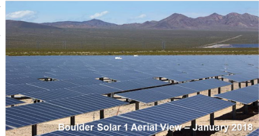
Boulder Solar 1 Ground View – January 2018
