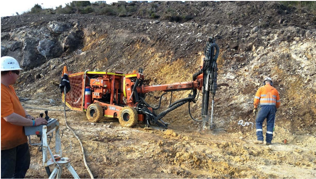
Figure 1 – Temporary site drill undertaking works for first bench blast at Granville East Mine
