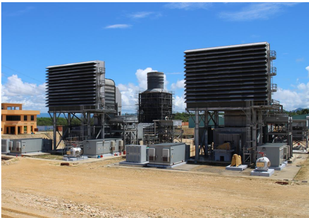
Pagbilao Power Plant
