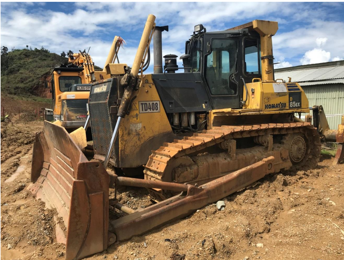
One of the 2 Komatsu D85 bulldozers put into operation during the Quarter
