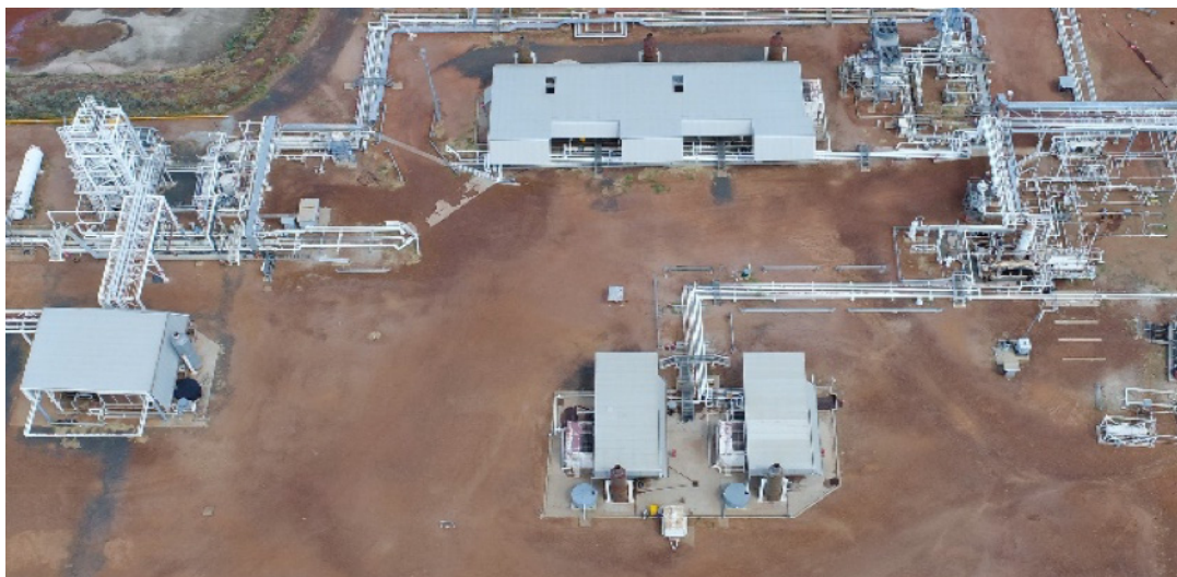
FIGURE 4 Kincora Gas Plant
