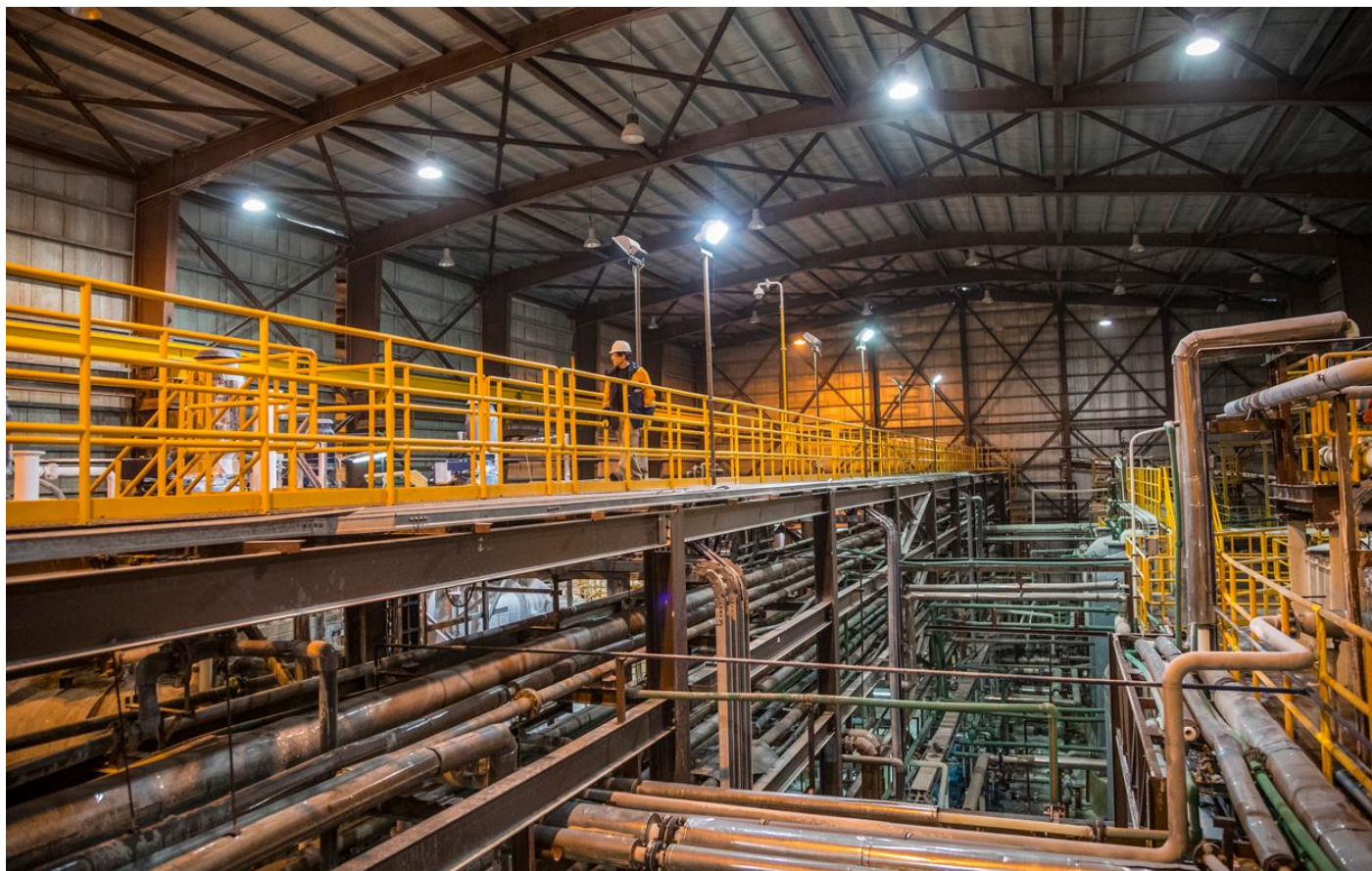
Olaroz Lithium Facility
