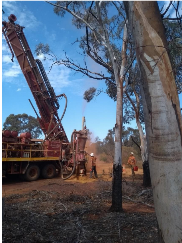
Figure 2: Reverse circulation drilling in progress on M27/263 at Silver Swan North during September 2018
