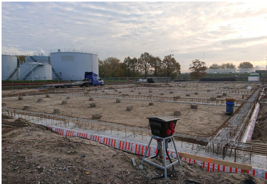
Photo of Amsterdam site showing concrete filled reinforced trenches and excavated pile tops ready for the concrete slab.
