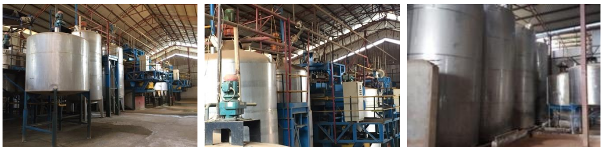
Figure 10, 11 and 12: The Luapula Processing Facility Precipitation Section
