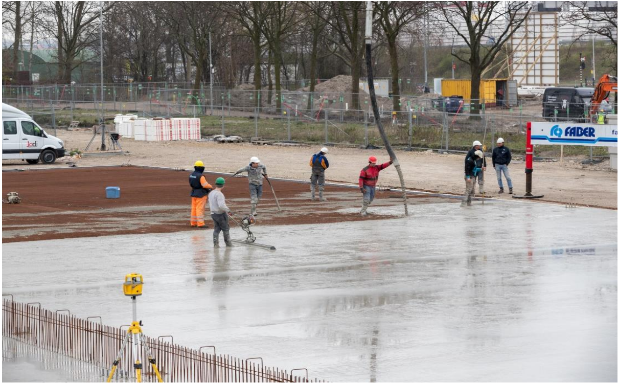
The final section of the production slab area having concrete poured into the steel mesh previously installed
