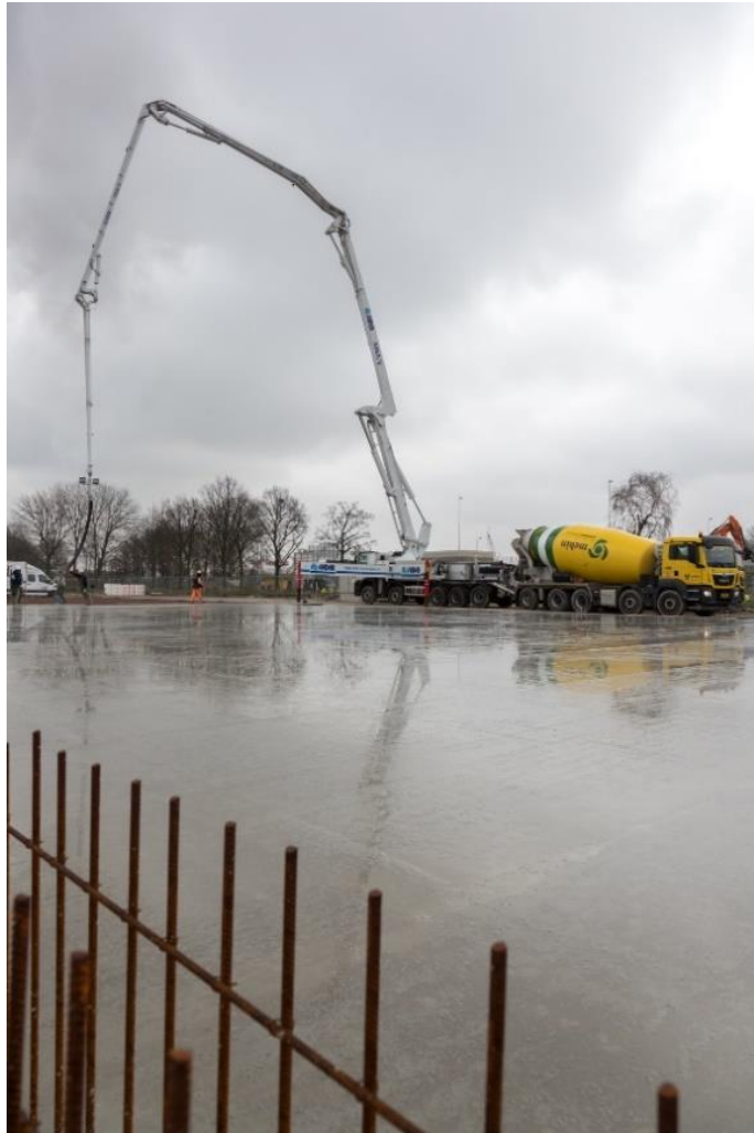
A total of 1,570 cubic metres of concrete was poured into the production slab.
