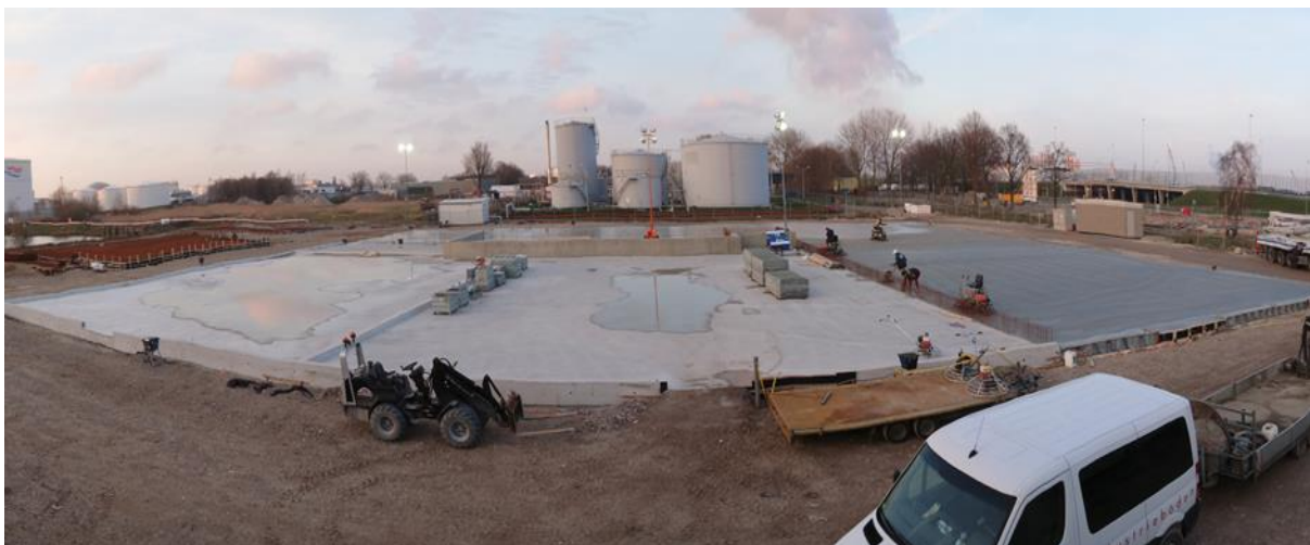
The completed concrete slab is 3,924 square metres in size. This photo shows the area that will support the production building on the left and the pre-production area on the right-hand side.
