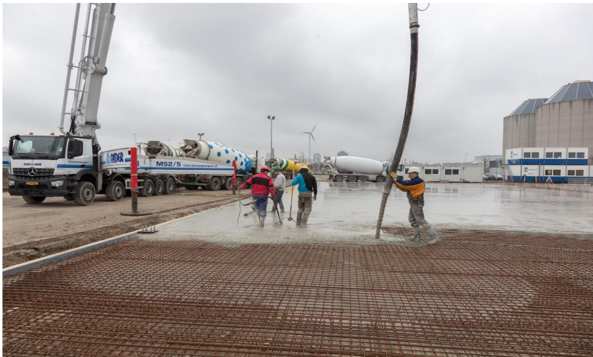
The concrete pour into the steel mesh previously installed in the production slab area which will support the IGES module
