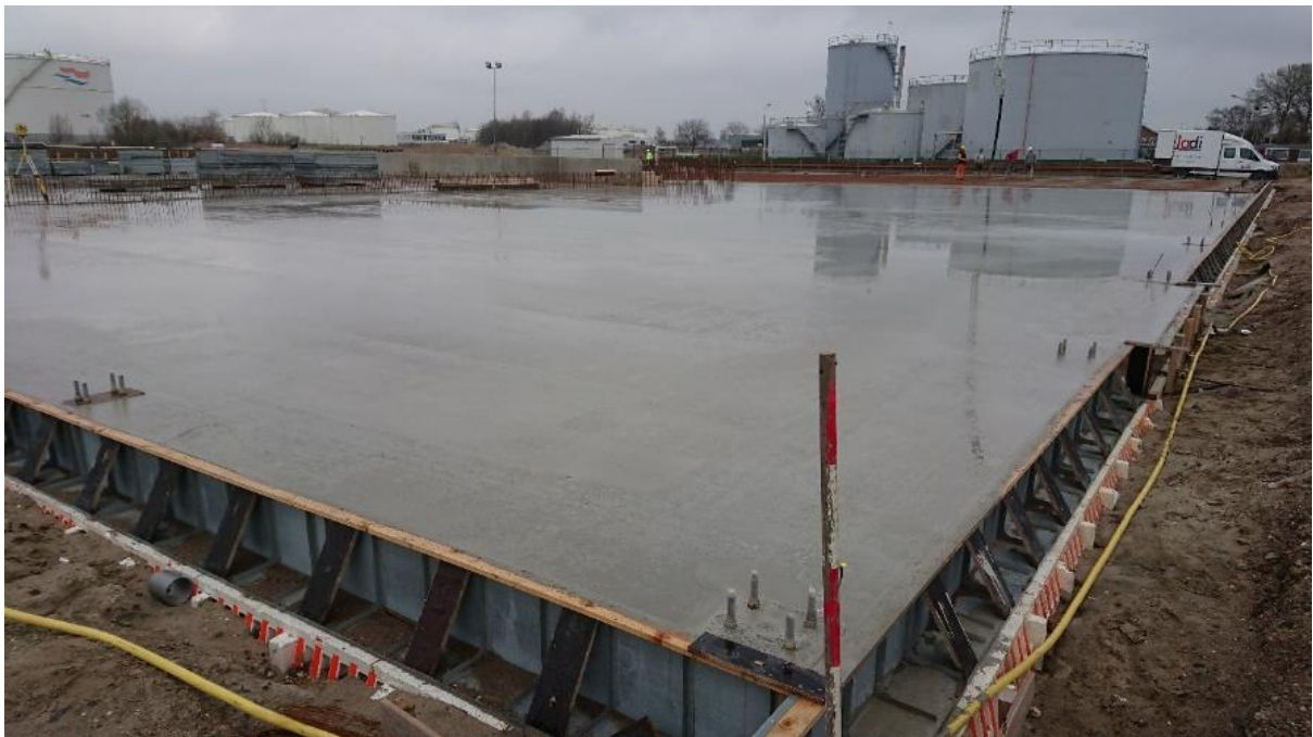
The freshly poured concrete slab that will support the production building and the IGES modules, photographed as it cures.
