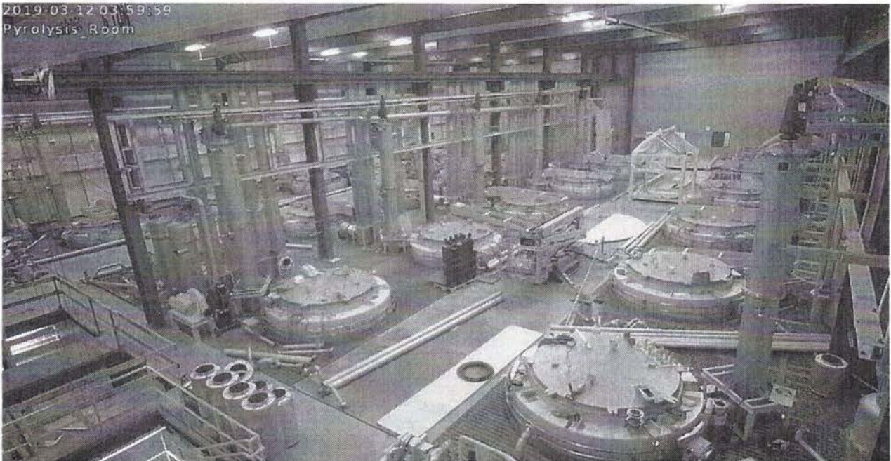
The Pyrolyx production facility under construction in progress in Terre Haute, Indiana (USA) March 2019
