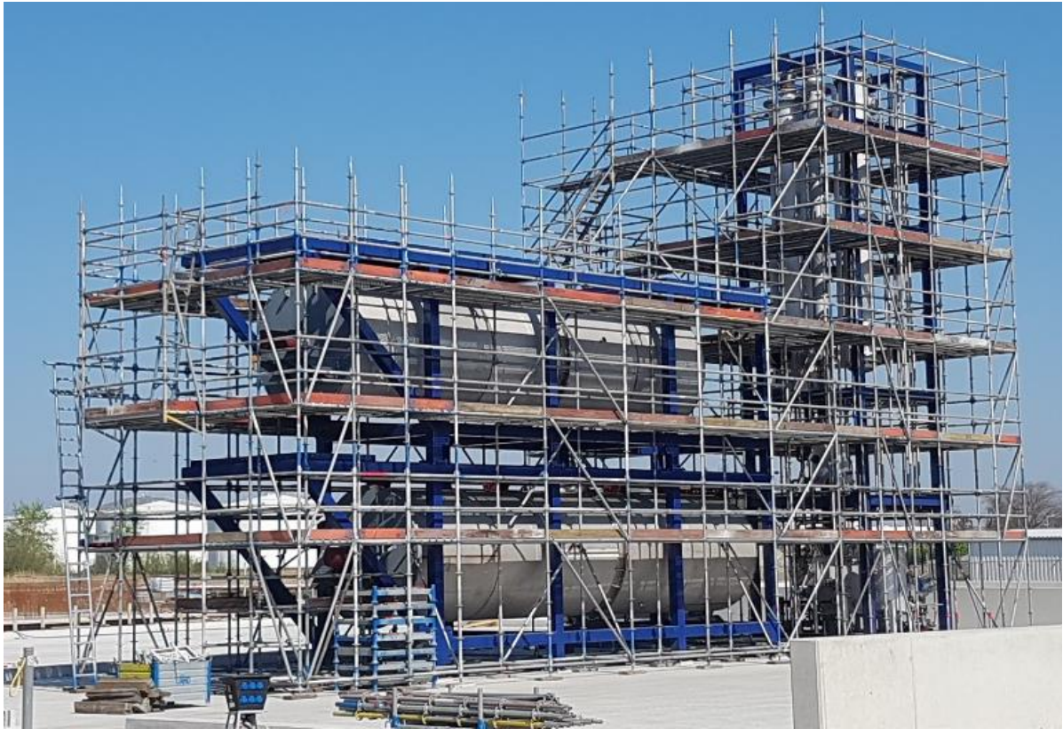
Module as installed in Amsterdam with scaffolding in place for ancillary equipment installation
