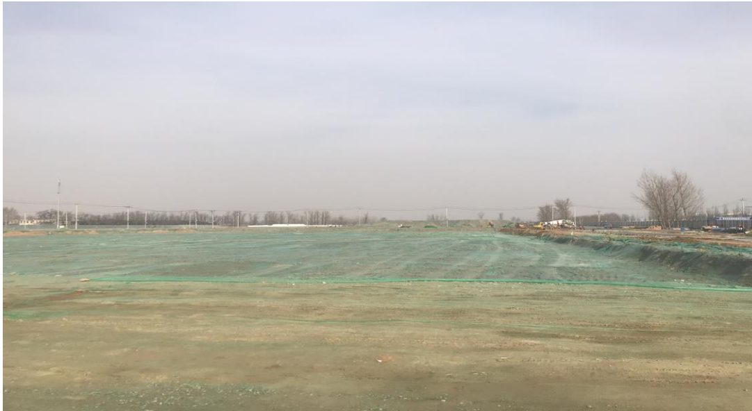
Part of the Beijing Wetlands Project site prior to the laying of a large geo-textile cover
