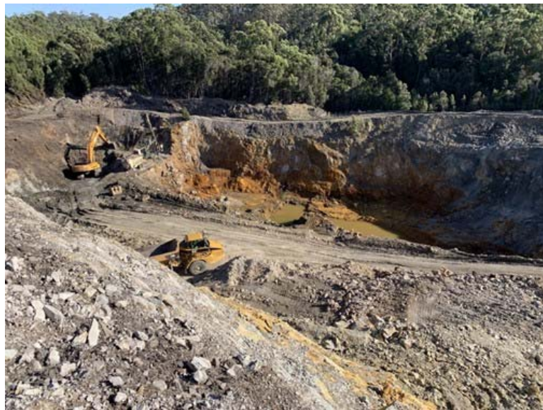
Figure 1 – Overview of open cut pit with skarn material (orange) in current base of pit (16 th April 2019)
