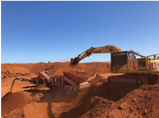
Figure 10: Screening into cement & fertiliser grade products
