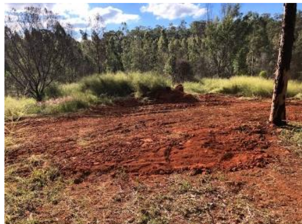
Figure 5: repaired site of pits BJP002 and BJP003 on old track in scrubland that had been burnt last year.
