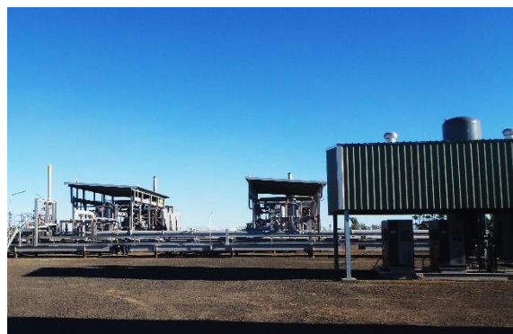
Compression equipment and pipe rack
