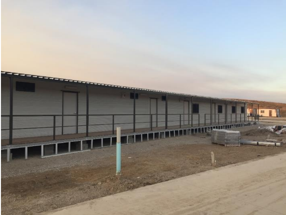
Recycling Amenities Building
