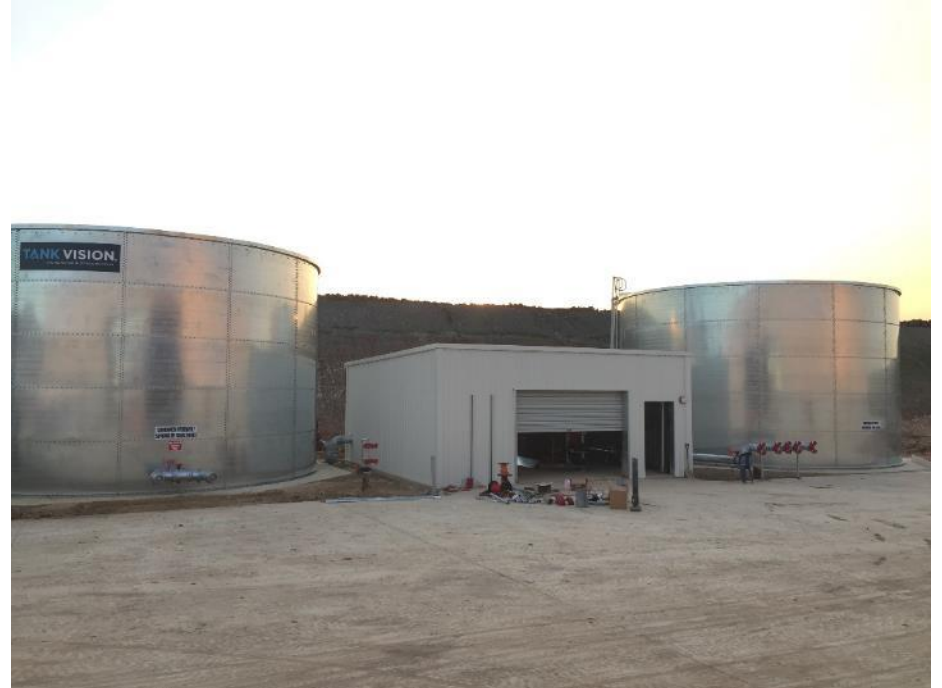
Fire protection water tanks
