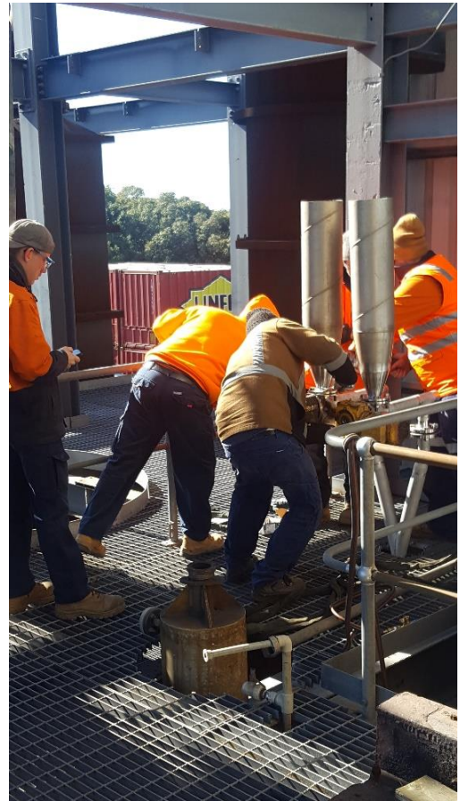
Installation of the hoppers for pellets and coal which is fed into the FB Roaster via double-dump valves
