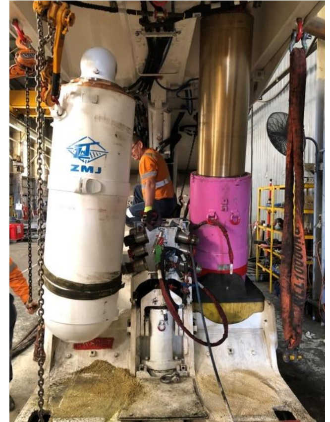
Mockup Prototype Leg Cylinder being trial fitted into existing spare Roof Support
