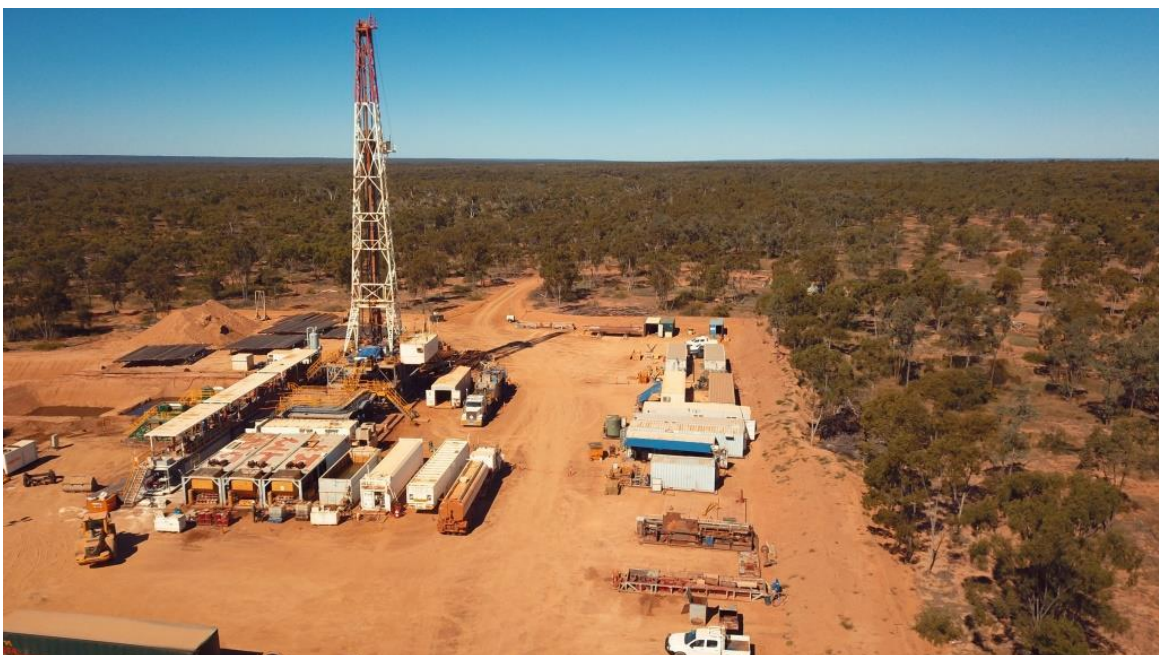
Figure 1: Ensign Rig 932 at Albany-2
