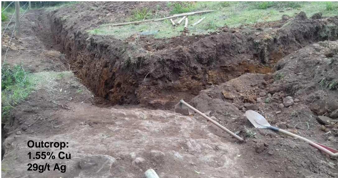
Figure 7 Trench Dug at Passo Feio Target cutting the Hydrothermally Altered Conglomerate that returned 1.55% Cu and 29g/t Ag
