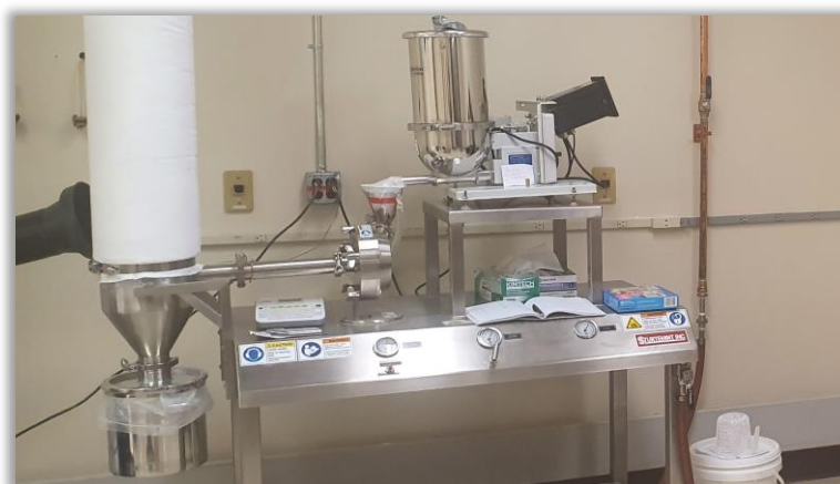
Alpha's dedicated Jet mill installation – Binghamton, USA
