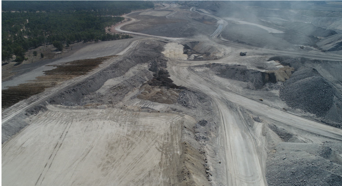
CHPP and ROM Area, with Rehabilitated Tailings Dam (post-mulch application) in the background
