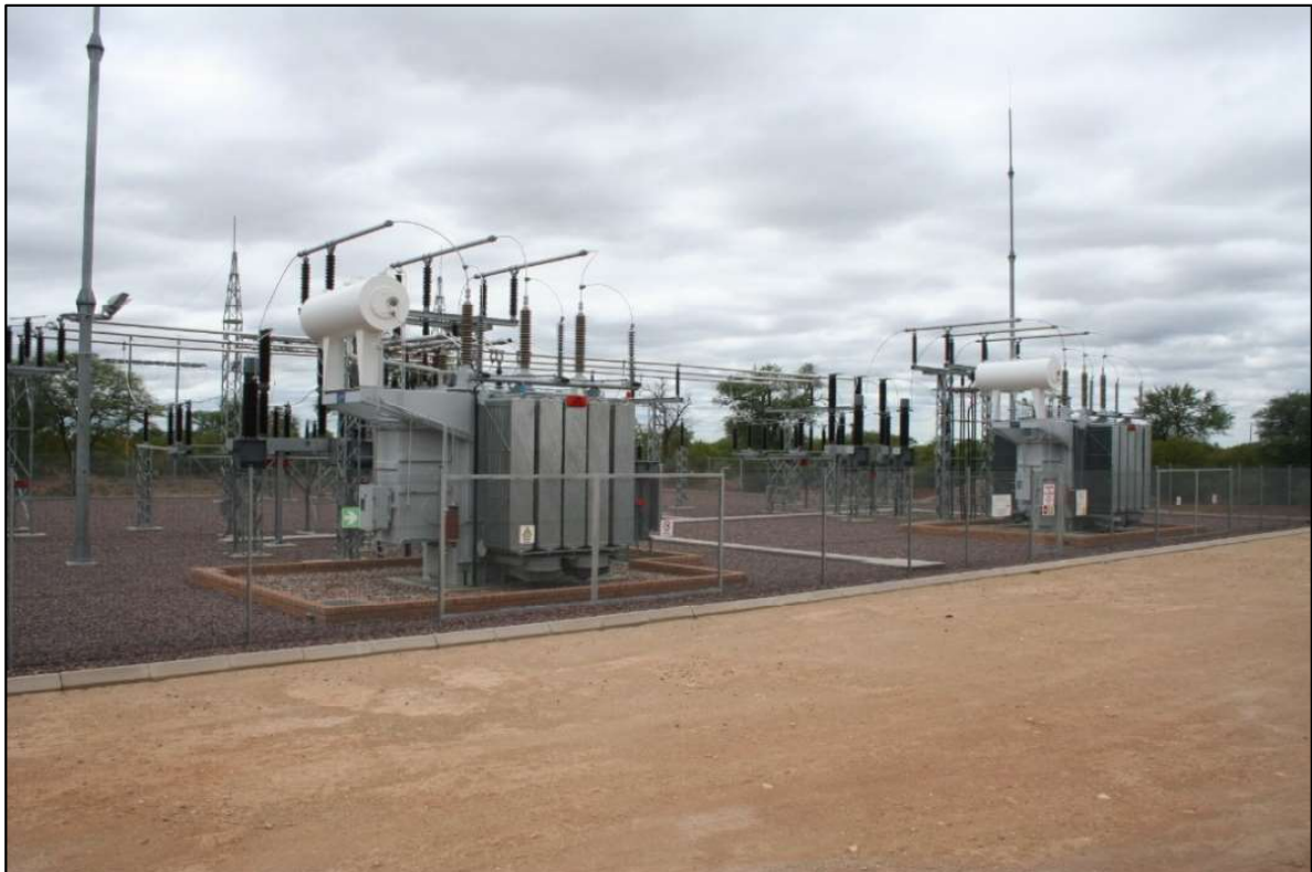
Figure 6-1: Electrical substation established at the Project
