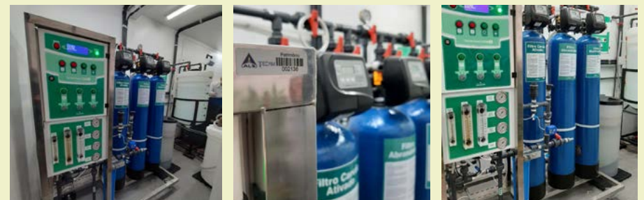
Life Sciences, Sao Paulo. Water purification system
