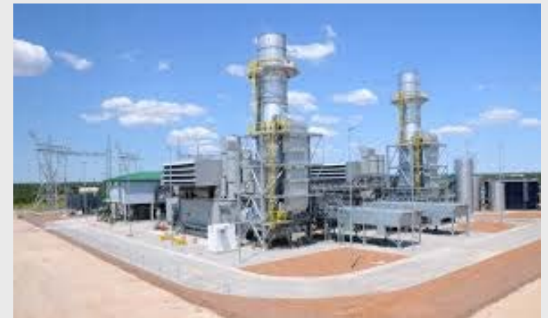
Orapa 90 Mw dual fuel power station
