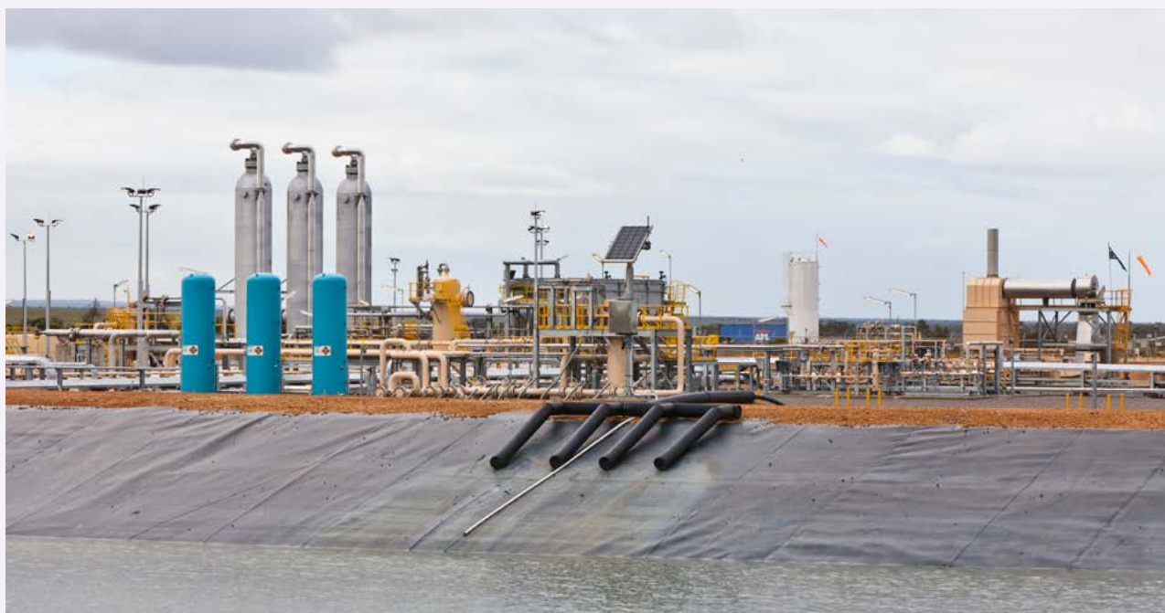
Mondarra Gas Storage Facility, Western Australia
