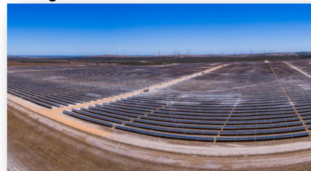
Darling Downs Solar Farm
