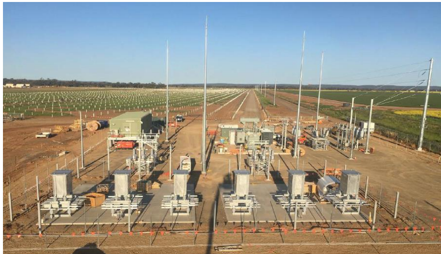
Figure 1. Jemalong Solar Project Substation Site
