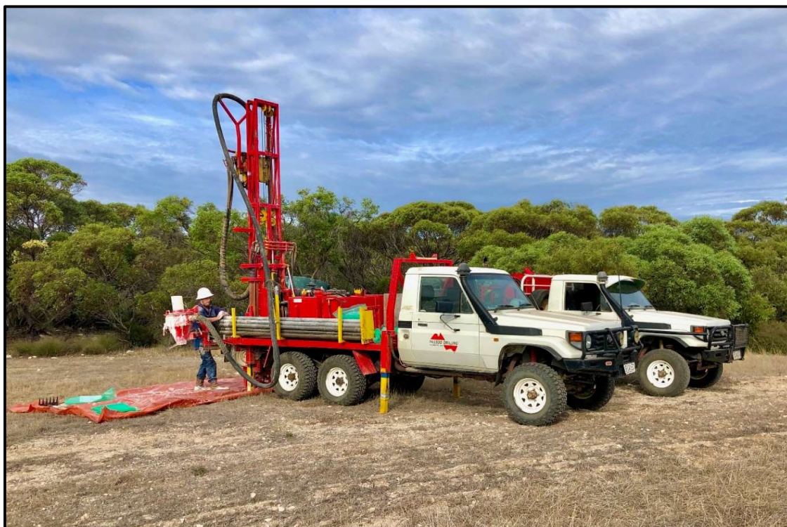
Figure 1: Air-Core Drill rig scheduled to mobilise to Gibraltar Project (EL6506), site 1 st week of November 2020
