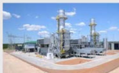
Orapa 90 Mw dual fuel power station
