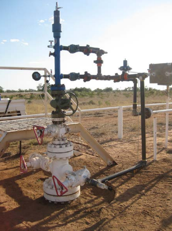
Carbean #1 with Successfully Installed Artificial Lift
