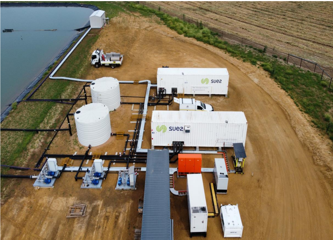
Figure 6 – Reverse osmosis treatment plant.
